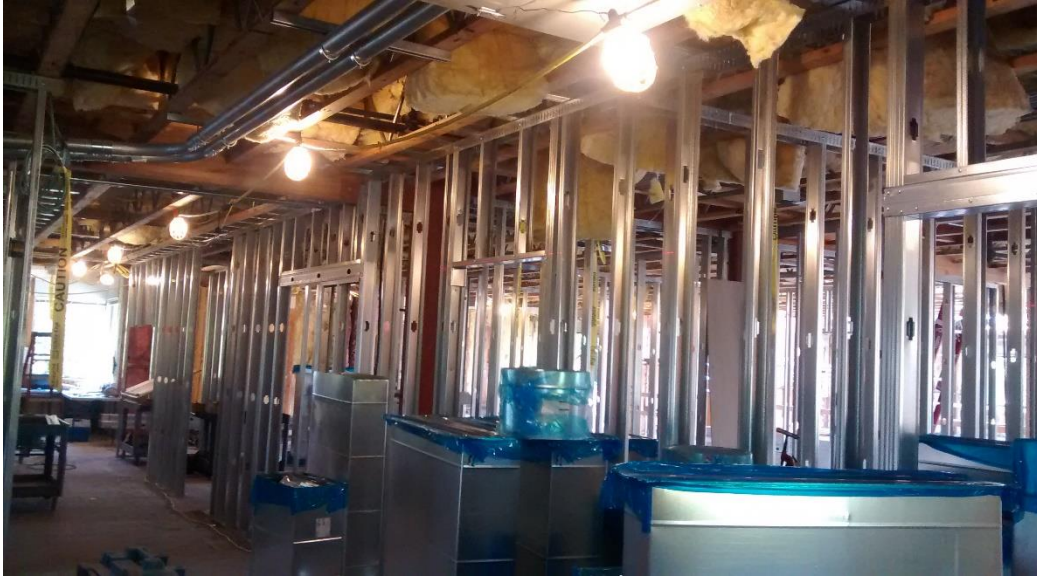
Figure 7-7 – Parallel fashion of work; wall framing, electrical, and duct install are nearly simultaneous due to crew sizes and space availability
